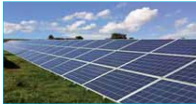
ET Solar connected a 2.65MW PV plant to the grid in France in October 2011.
