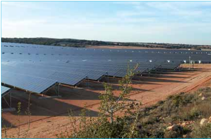
Figure 1. View of a 10MW utility-scale PV installation in Osa de la Vega, Spain.
