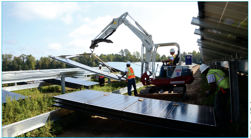
Figure 2. Delivery of preassembled racking and modules to the site for installation (the North Carolina Progress Energy II project).
