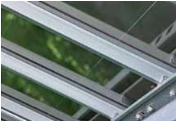
Backside of on-site-bonded PV modules as part of a greenfield PV installation.
