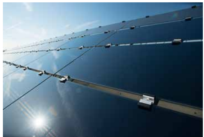
Credit: First Solar
