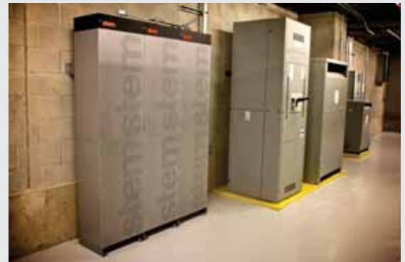
Stem is installing commercial-scale battery storage units under a contract with Southern California Edison.
