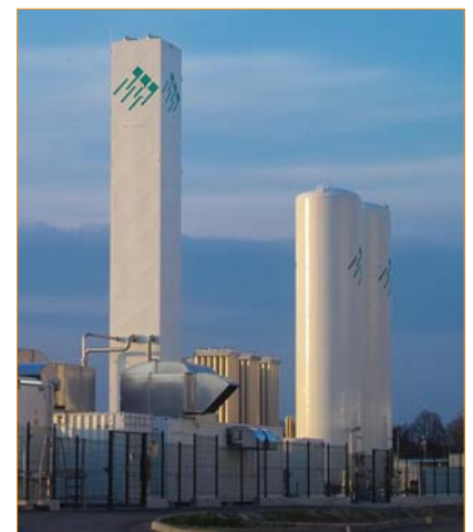
Figure 7. On-site nitrogen generation (courtesy of Conergy AG).
