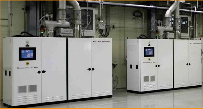
Figure 8. On-site fluorine generation.
