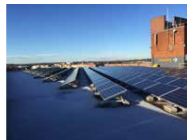
South facing system on flat roof
