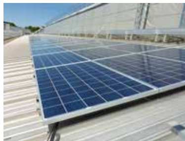
Flat-to-roof system on South/East/West pitches
