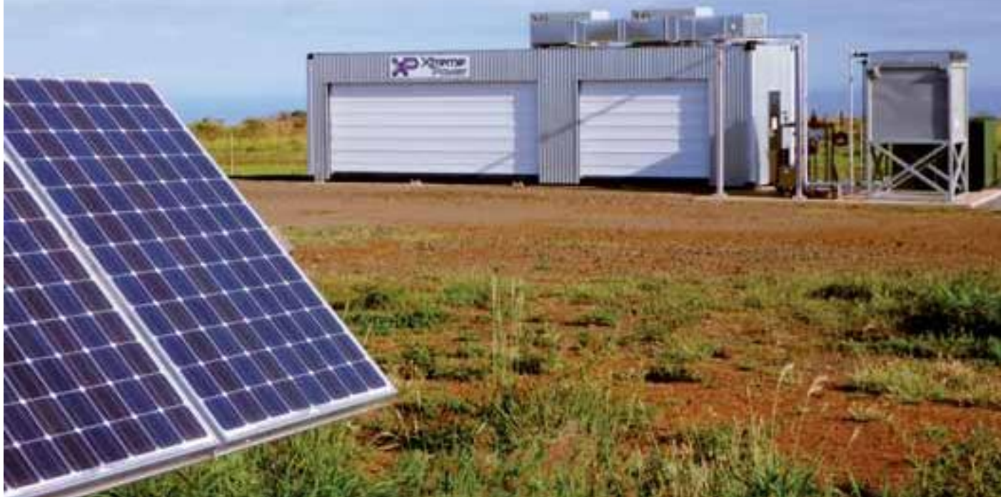
Xtreme Power's storage facility on Lanai, Hawaii, is used to double the output of solar and control ramp rate.
