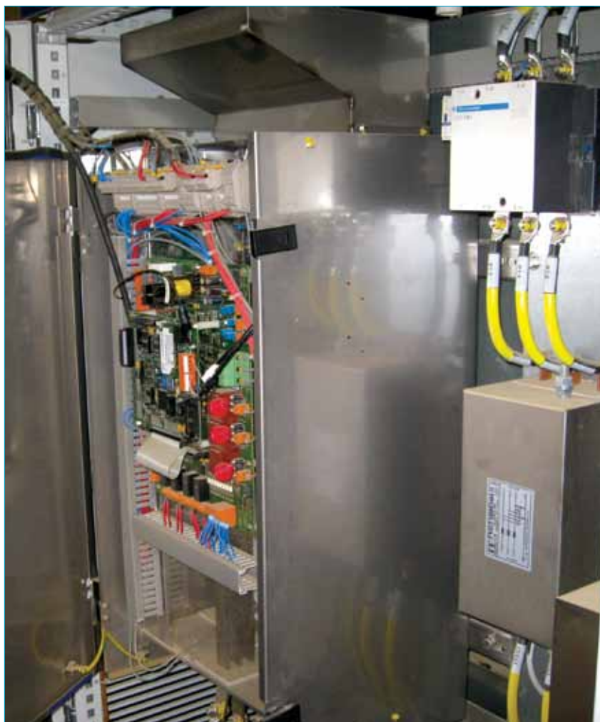
Figure 1. A PV grid-connected inverter installed in a Spanish PV plant.
