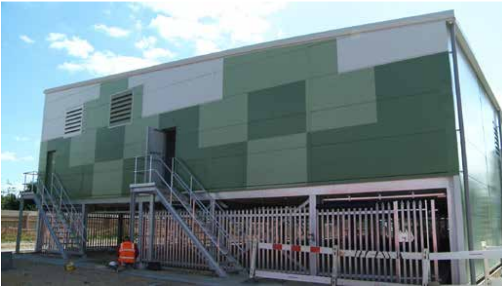
Credit: S&amp;C Electric
