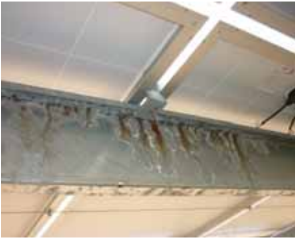
Figure 1. Oxide on a structure as a result of insufficient galvanising.
