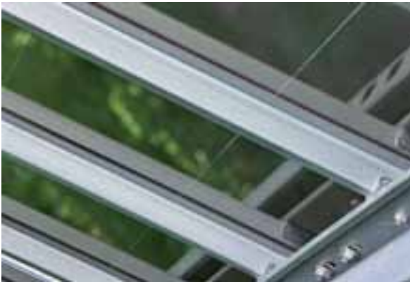
Backside of on-site-bonded PV modules as part of a greenfield PV installation.
