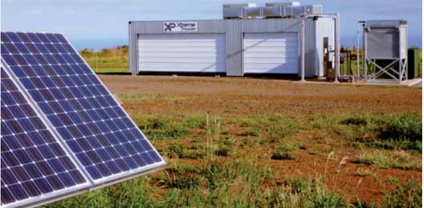
Xtreme Power's storage facility on Lanai, Hawaii, is used to double the output of solar and control ramp rate.
