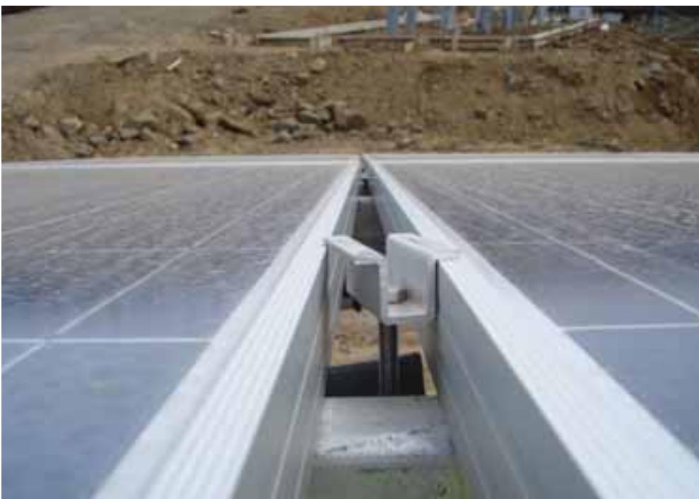
Figure 2. An incorrectly installed omega junction.
