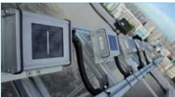
▼ Figure 4. The irradiance measurement station located on the roof at the Solar Energy Research Institute of Singapore (SERIS).
