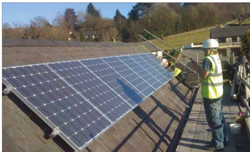
Figure 3. Integrated solar PV on a new build domestic home in south Scotland.
