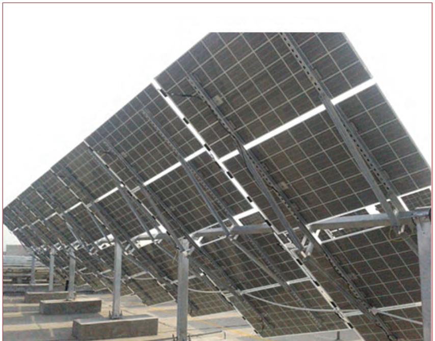
Figure 3. Example of a PV system using BYD's double-glass modules.
