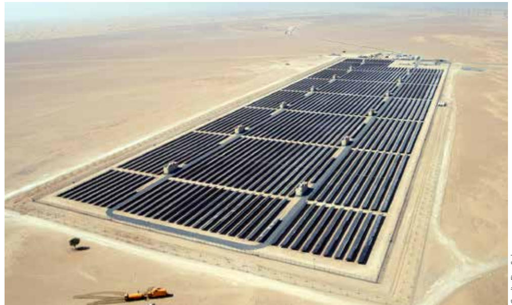
Credit: First Solar
