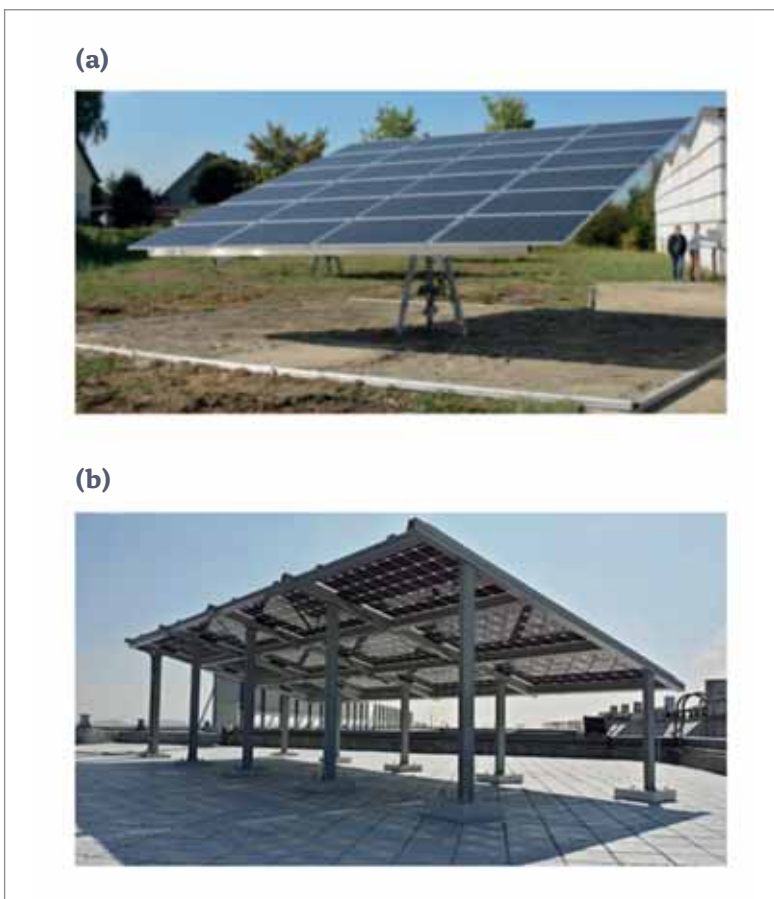
Figure 4. Field installations of bifacial modules using PERC+ solar cells: (a) 13kWp Bisun modules from SolarWorld mounted on a single-axis tracker system [27]; (b) 2MWp rooftop installation currently under construction by Neo Solar Power, implementing their Glory BiFi modules [29].
