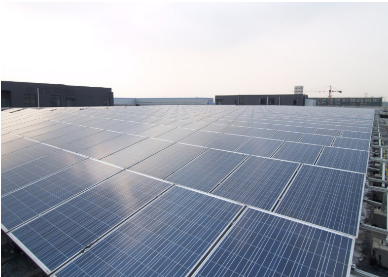
Figure 6. PV installation on a commercial building
