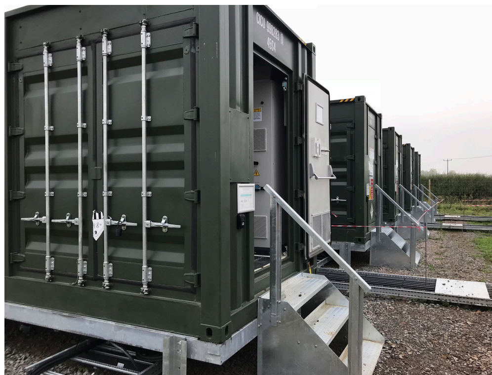
Battery systems sitting alongside solar projects, such as the UK's Clayhill, will become more common as storage plays an increasingly important role in grid balancing
