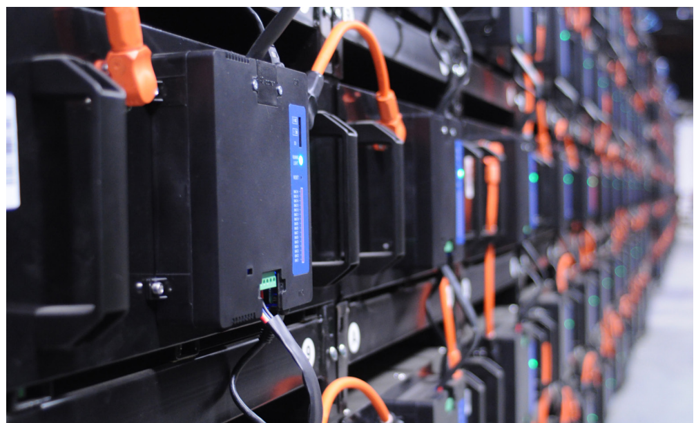
Credit: Powin Energy
