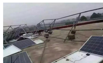
Failure caused by poor mounting structure design
