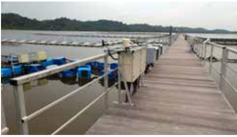
Figure 11. Meteorological station on the floating pontoon
