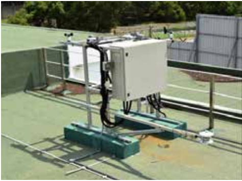
Figure 10. Meteorological station at the rooftop
