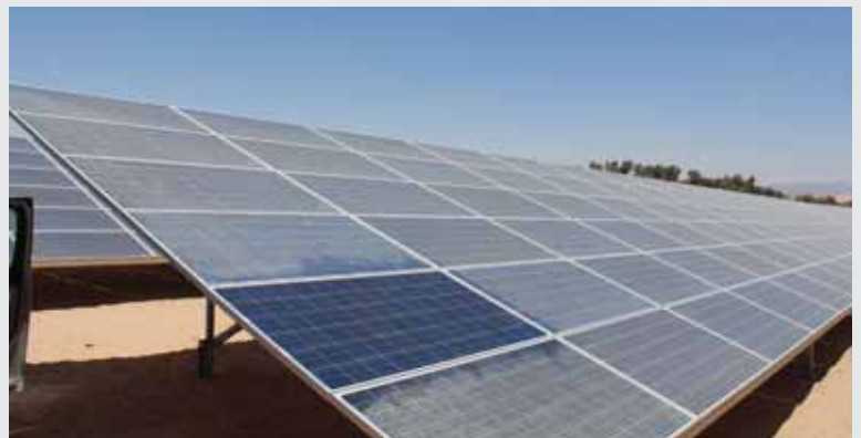
Standardised testing procedures are helping shed light on the impact of cleaning technologies on module performance
