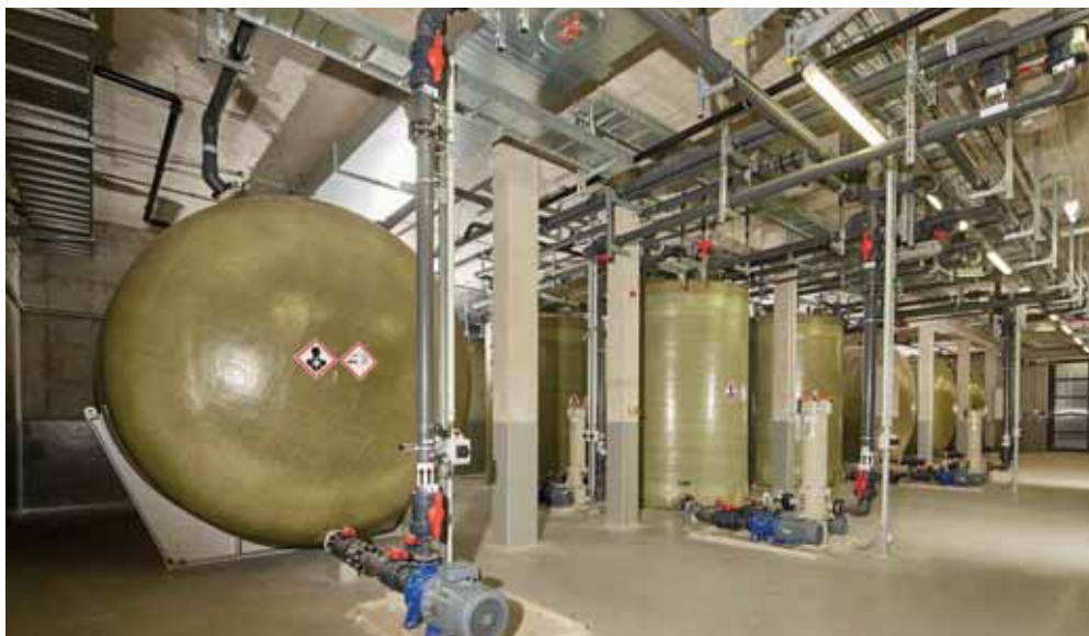
Tanks of a 2MW/20MWh vanadium redox flow battery at Fraunhofer ICT
