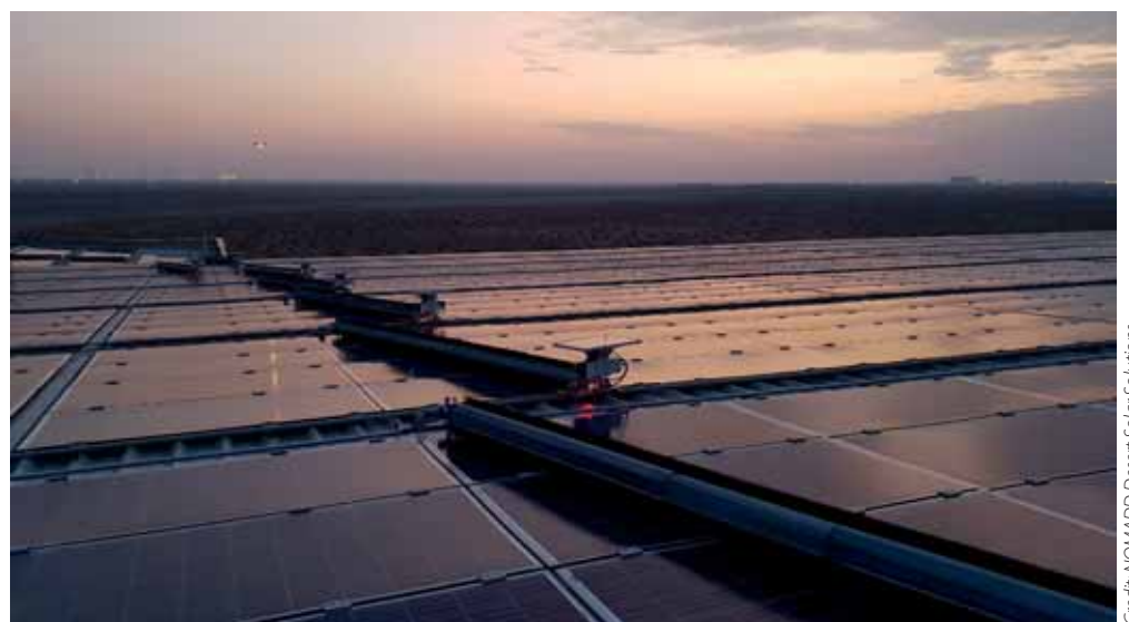
Figure 8. Dry-brush automatic cleaning machines are gradually being deployed at commercial PV projects in desert regions.
