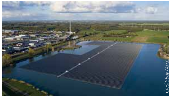
The recently completed 14.5MWp Sekdoorn plant in the Netherlands was designed to optimise the levelised cost of electricity, according to developer Baywa r.e.
