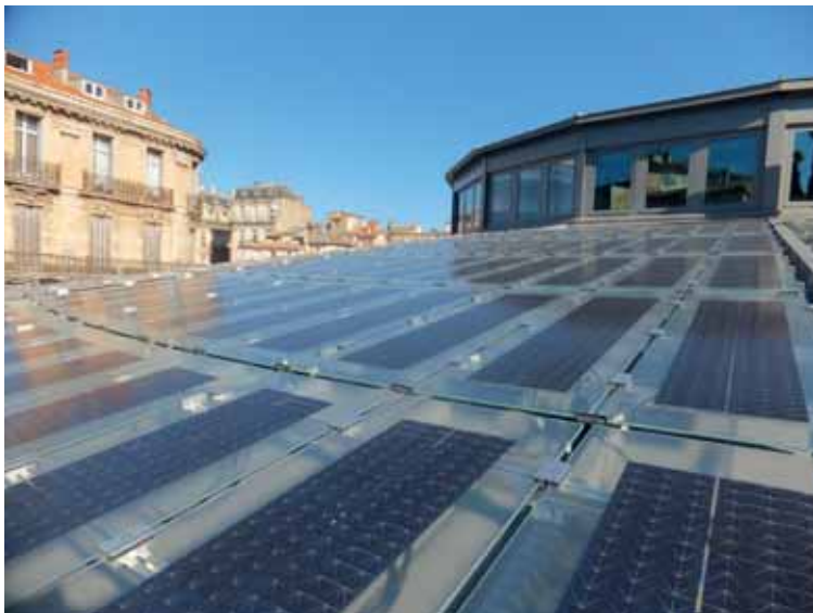
▲ 990 modules have been installed with an estimated Power of 65kWp; they show a tetragonal shape with five different dimensions to fit the circular area of the roof
