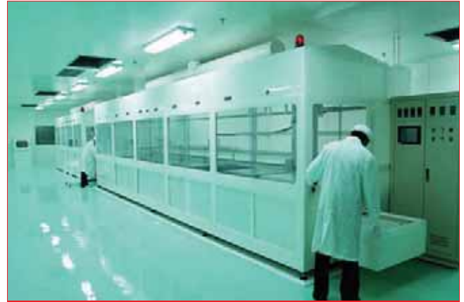
Washer line at Solar EnerTech's production facility.
