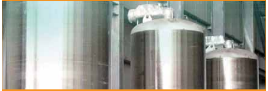
Deposition reactors at Hoku's Pocatello, Idaho polysilicon manufacturing facility
