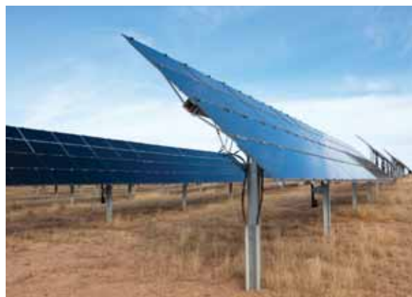
Credit: First Solar
