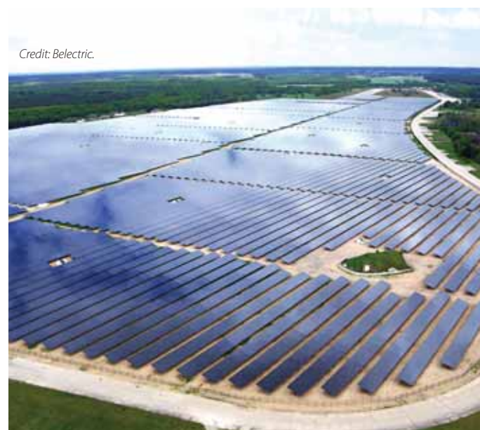
The Alt Daber power plant in Brandenburg, Germany.
