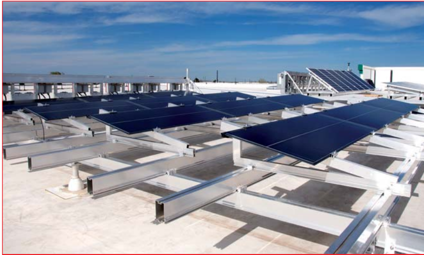
ProLogis' 11kW (DC) rooftop module test system, Denver, CO.
