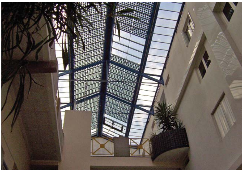
Figure 2. BIPV installed on a glass roof.
