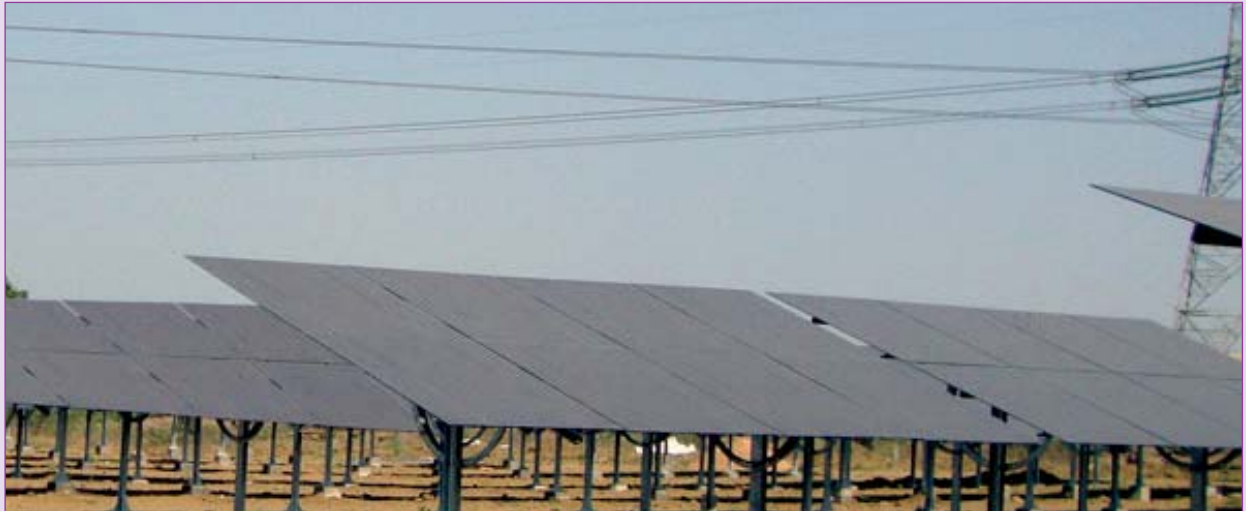
Moser Baer's 1MWp field installation in Maharashtra, India.
