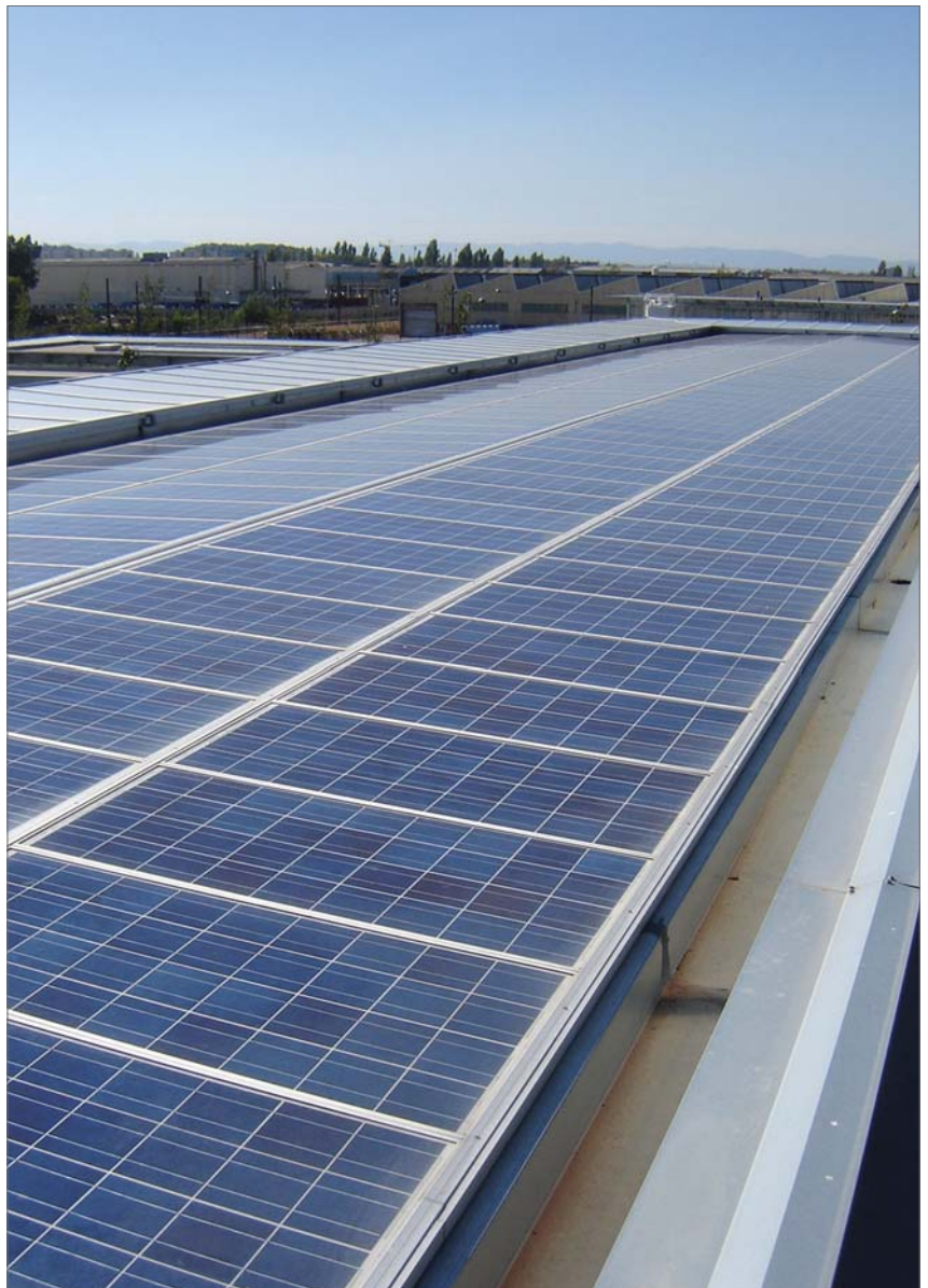
Figure 1. BIPV installed on an industrial roof.
