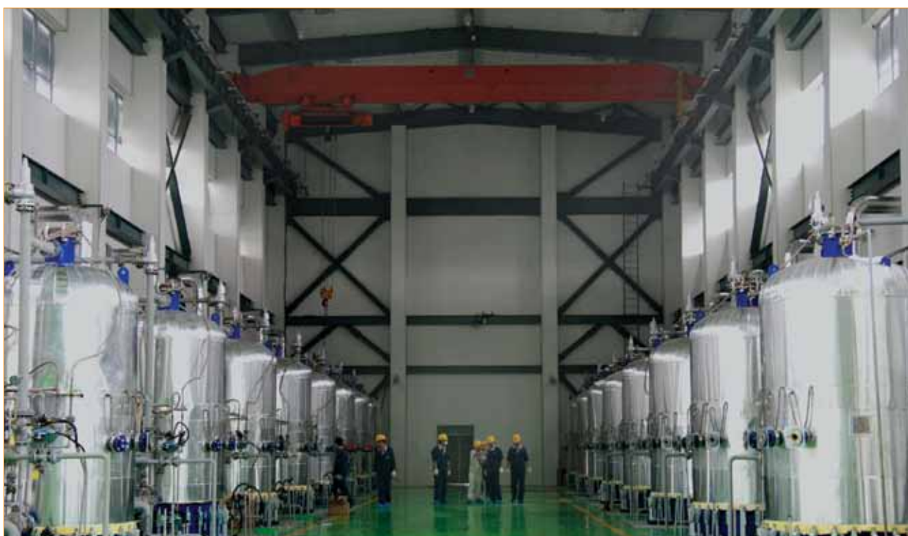
Figure 3. CVD reactors in the polysilicon plant deposition building.
