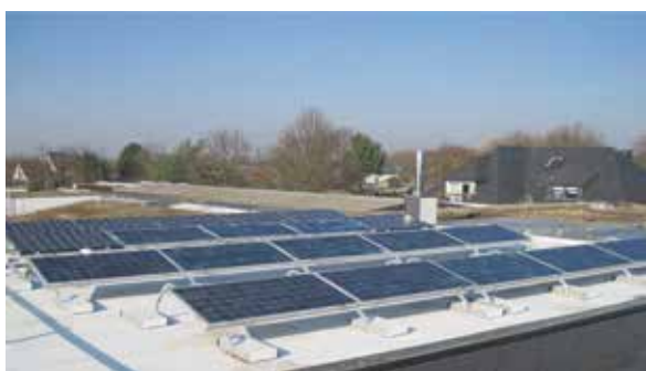
Figure 10. Rooftop test field in Geilenkirchen
