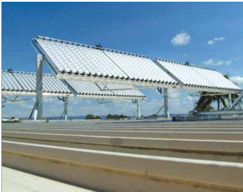
Figure 7. Whitfield Solar's WS:Si24 solar concentrators installed on a residential rooftop in Queensland, Australia.
