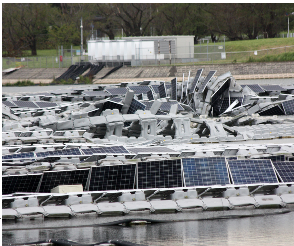
Figure 5 Typhoon caused fire on Japan’s largest floating PV site on Yamakura Dam in 2019
