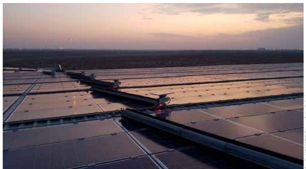
Figure 8. Dry-brush automatic cleaning machines are gradually being deployed at commercial PV projects in desert regions.
