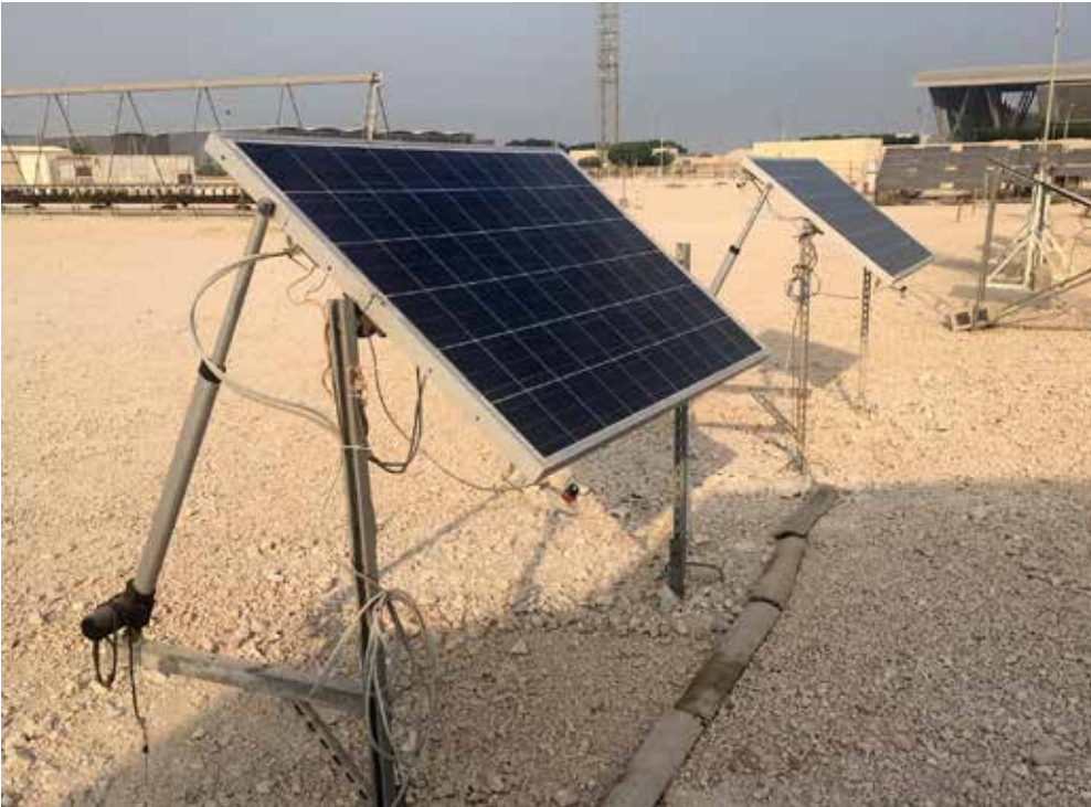
Figure 7. Test trackers with enhanced tilt ranges at the OTF in Qatar. Soiling was greatly reduced by vertical night stowing, but there was little gain from tilting to enhance dust resuspension during wind [13]
