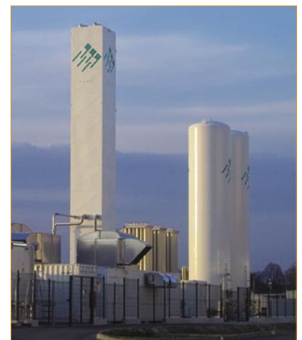
Figure 7. On-site nitrogen generation (courtesy of Conergy AG).
