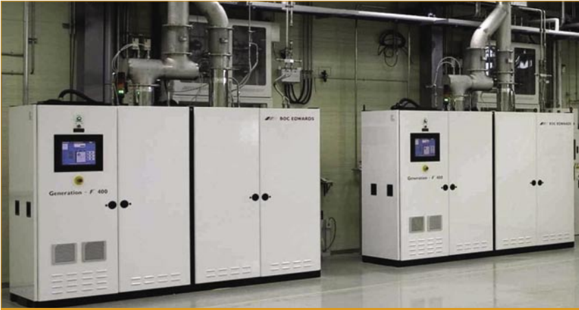
Figure 8. On-site fluorine generation.
