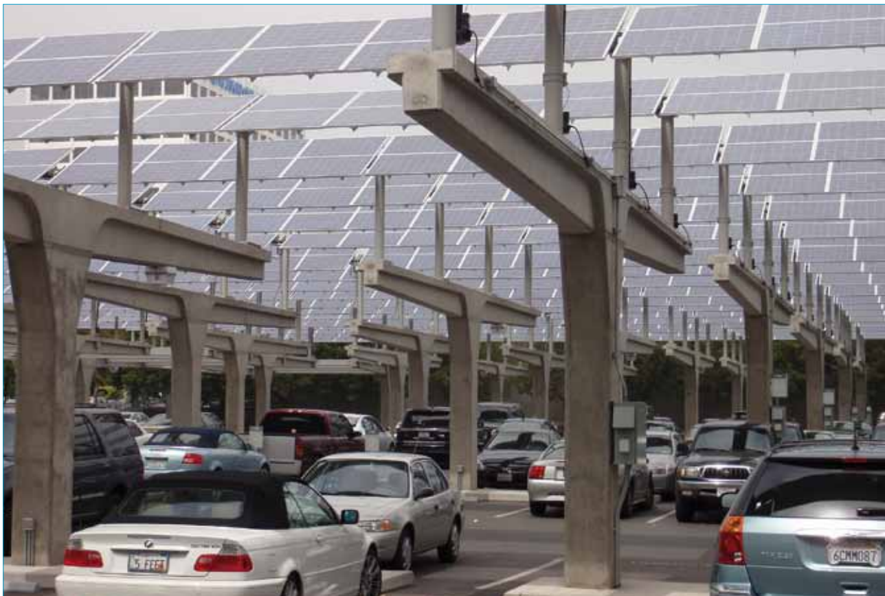
Figure 1. Photo of the tracking PV system installed by Raytracker, Inc. at the British Telecom US Headquarters, El Segundo, California.
