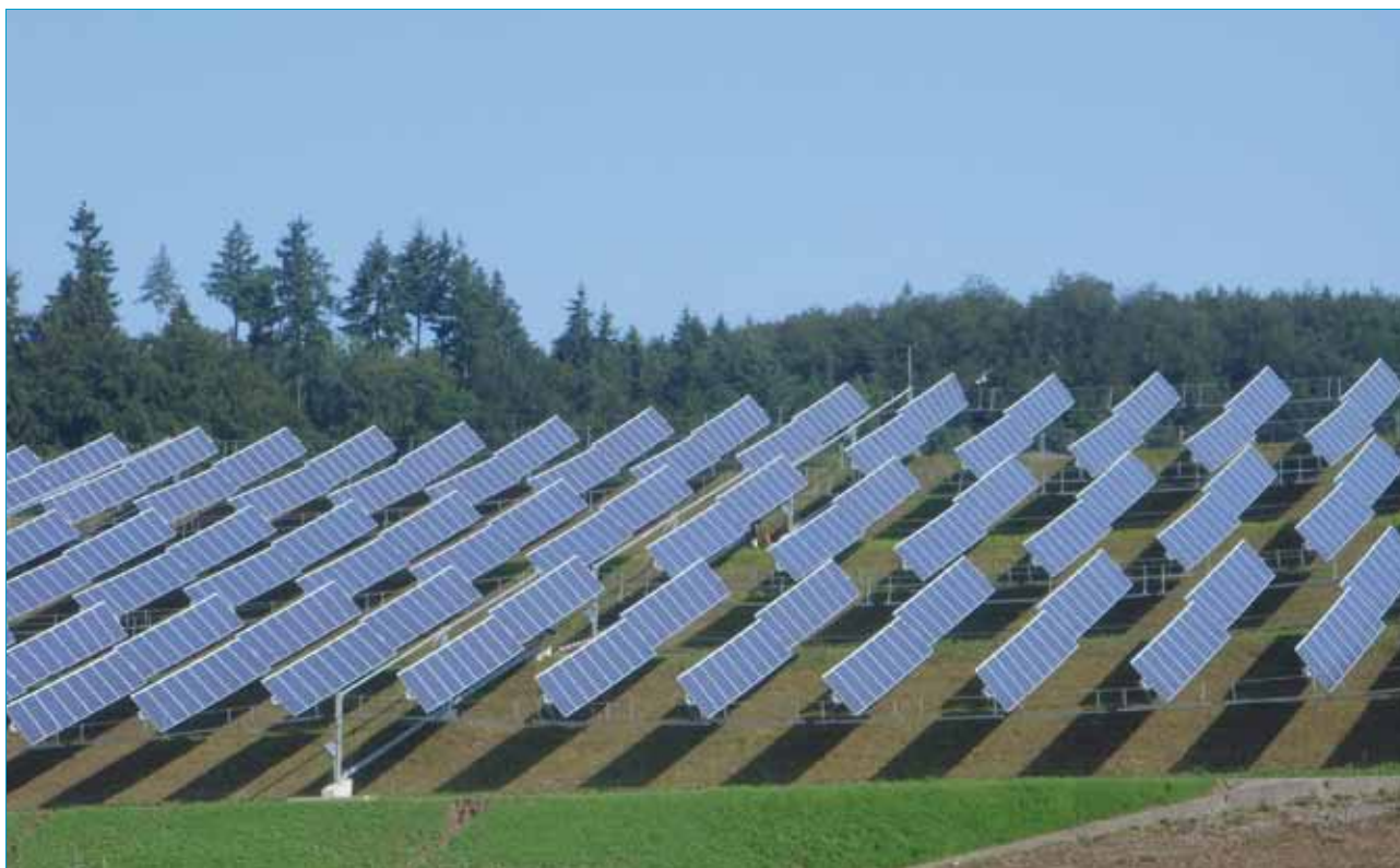
Figure 2. The Solar Wings PV installation. 647kWp of modules are mounted on a single-axis tracking system with the rotation axis aligned about 15° away from north/south towards southwest, and inclined 23° from horizontal.
