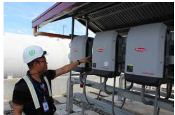
The project uses 60 Fronius inverters
