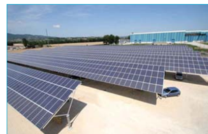
TerniEnergia installation using SolarWorld modules.
