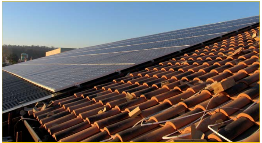
Figure 2. Example of BAPV roof installation.
