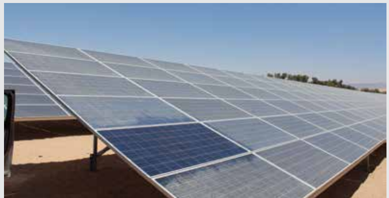
Standardised testing procedures are helping shed light on the impact of cleaning technologies on module performance
