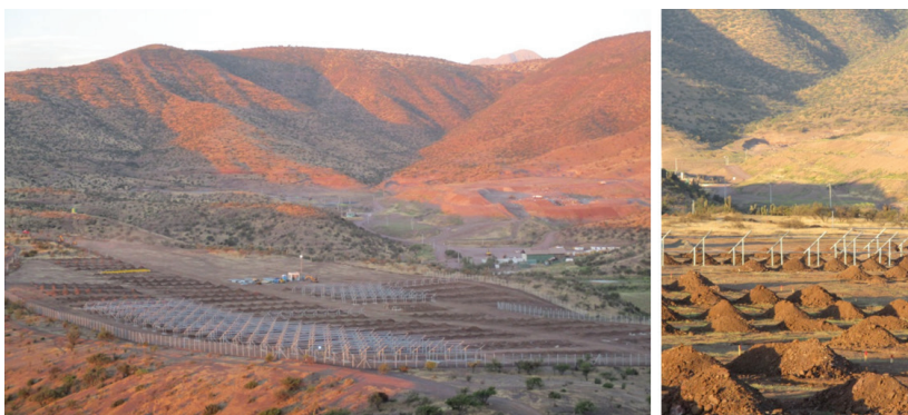
Figure 8. The bifacial PV system currently being set up by MegaEngineering and Imelsa. With a total power of 2.5MWp and 3.25MWpe [15], the 'BiSoN farm' will become the world's largest bifacial PV system.
