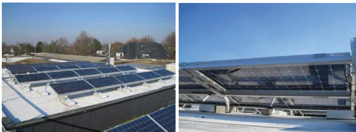
Figure 10. A commercial installation in Geilenkirchen, Germany, monitored by Fraunhofer/ISE (20cm height above the rooftop, 78% reflectance white roof membrane, nine-month period). Results: bifaciality gain = 21.4%; effective cell efficiency = 22.5% [13].v
