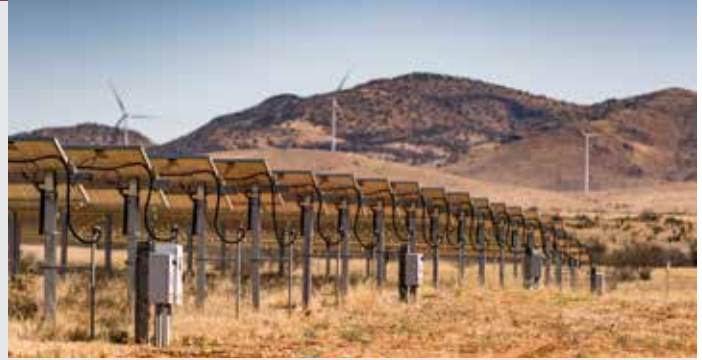
Credit: Swinerton Renewable Energy
