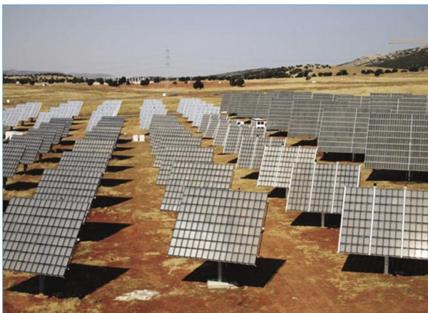
Figure 6. ISFOC HCPV power plants in Puertollano.
