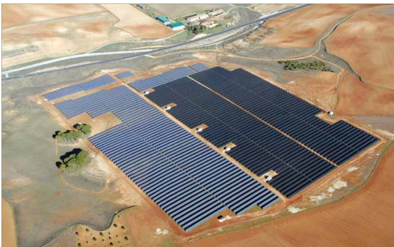
Figure 2. The Villanueva de la Jara PV power plant, Cuenca, Spain, consists of c-Si and CdTe modules, constructed by Phoenix Solar in 2008.
