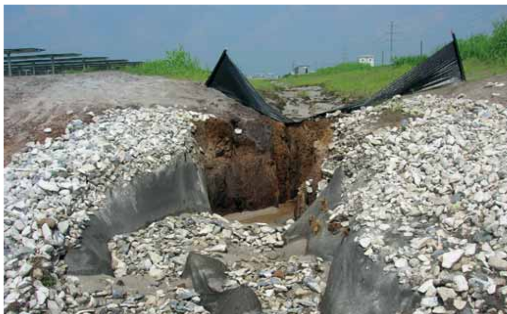
Proper installation of erosion control materials is critical for function during and after construction of PV power plant, particularly in regions with high rainfall
