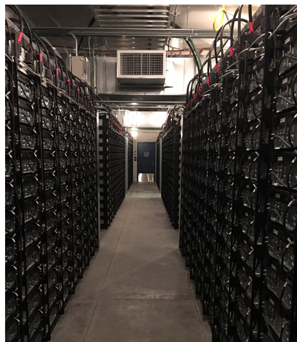
Credit: Greensmith Energy
