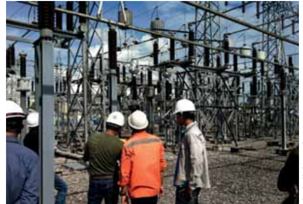
Thailand utility EGAT is looking at floating solar and storage.
