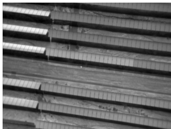
Figure 4. Disconnected string detected with aIRT on a single-axis tracking, utility-scale PV power plant
