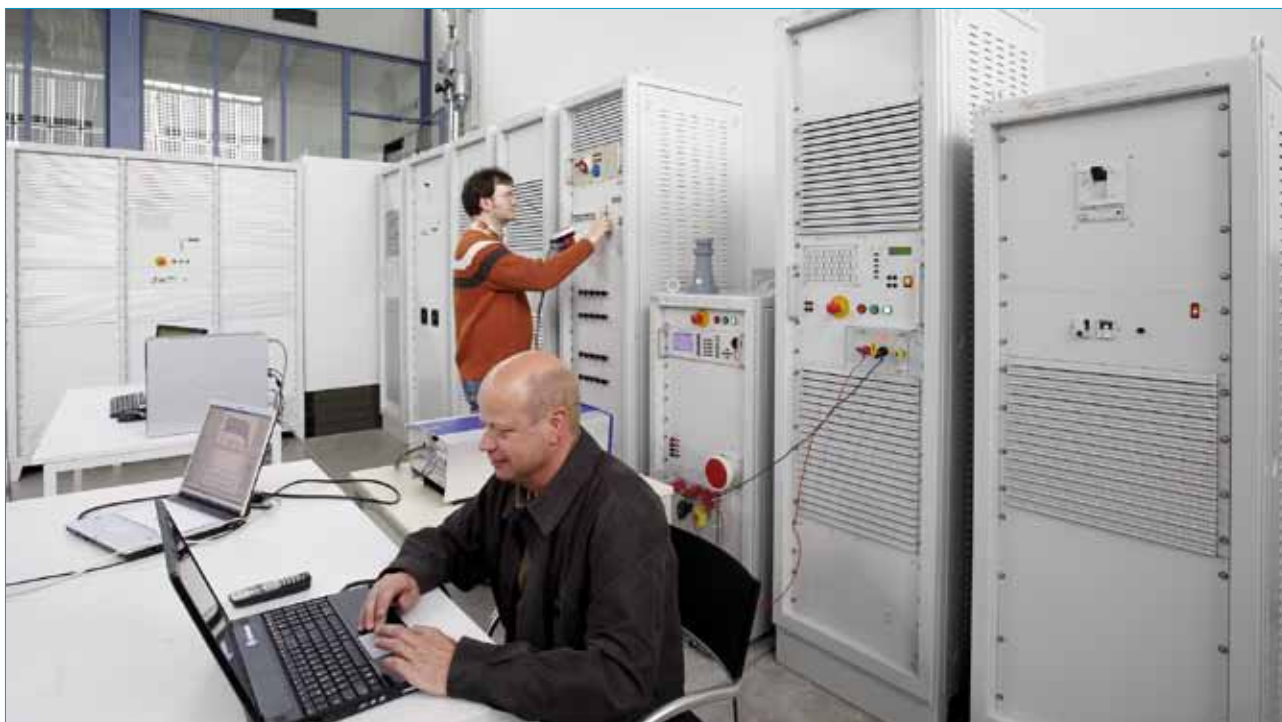
Figure 5. ISET's facility for PV inverters to test conformance with interconnection requirements.
