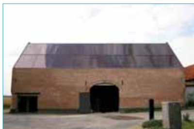
Gehrlicher's GehrTec Intra substructure allowed Masdar PV's 5.7m 2 thin-film solar modules to be fully integrated into the sloping roof of the 19th century barn.
