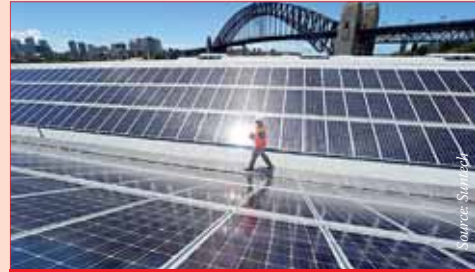
Suntech's Pluto technology, developed in collaboration with the University of New South Wales, has been installed in this project in Sydney, Australia.
