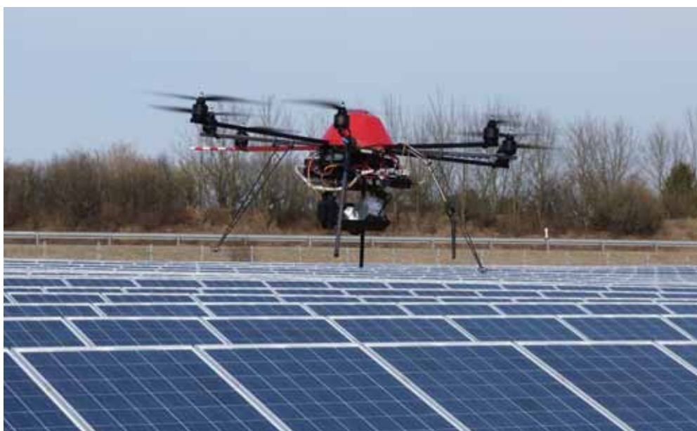
Figure 1. Inspection of an installed PV plant using an aerial, unpiloted IR-measurement system consisting of an octocopter with control unit, a fast and high-resolving IR camera and a visual camera for orientation.
