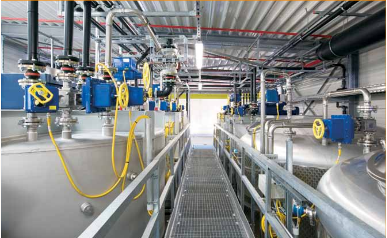
Figure 6. CRS Reprocessing Services' typical slurry recycling system.
