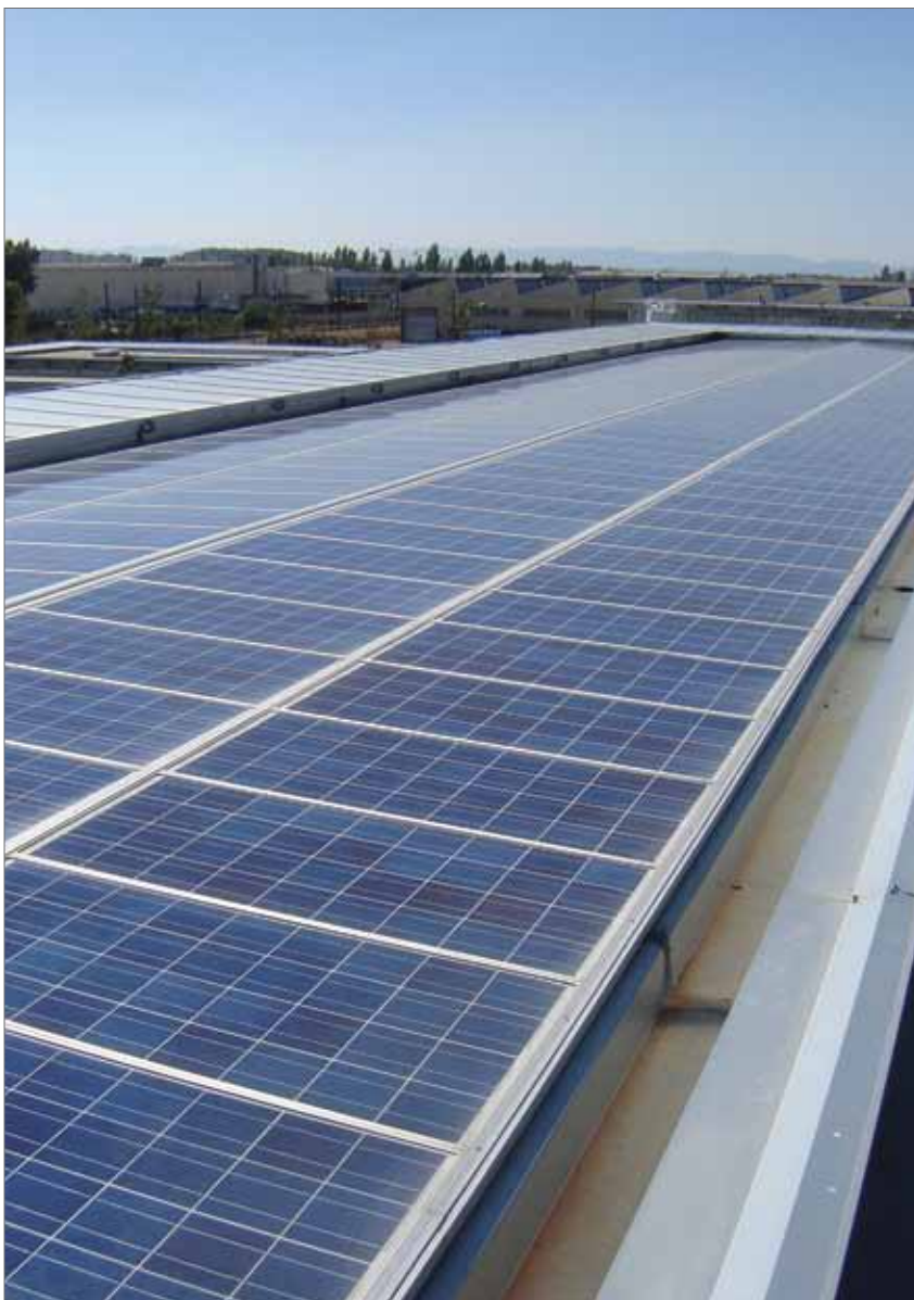
Figure 1. BIPV installed on an industrial roof.
