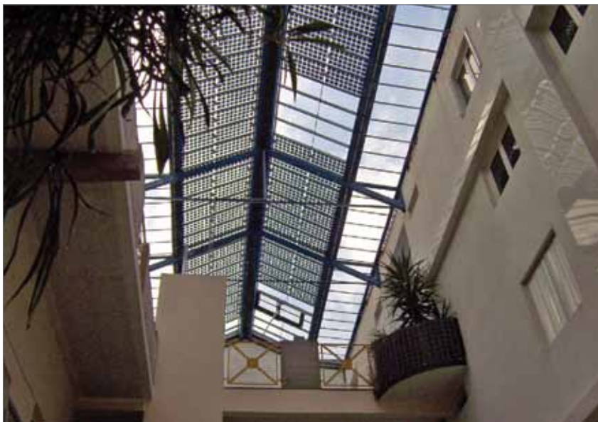
Figure 2. BIPV installed on a glass roof.
