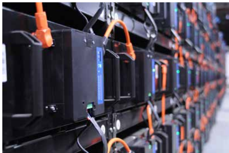
Powin Energy commissioned the 2MW/8MWh Grand Johanna storage facility within just a few months of being given approval for the project
