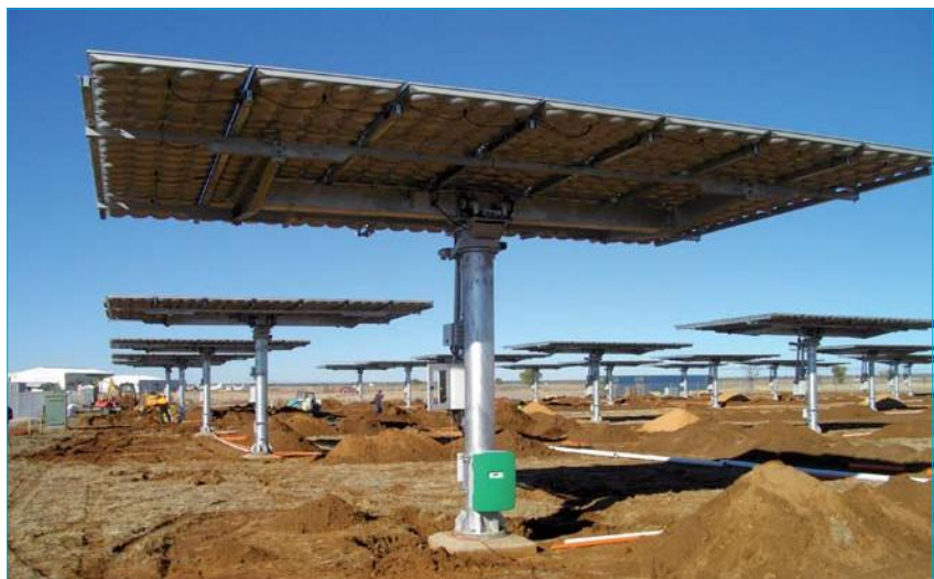
The Alice Springs Project in Australia features 235kW of CPV arrays.
