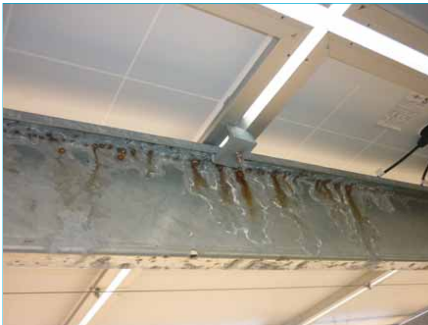
Figure 1. Oxide on a structure as a result of insufficient galvanizing.
