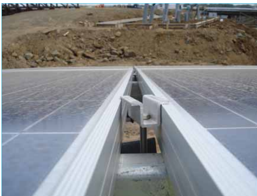
Figure 2. An incorrectly installed omega junction.
